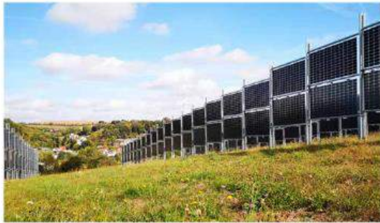
Figure 35: Bifacial modules installed vertically, Donaueschingen. © Next2Sun GmbH
